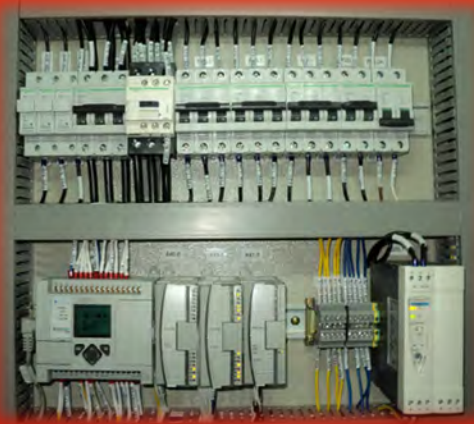
Control With AB PLC
