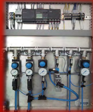
Electrical with Pneumatic Control
