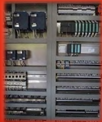
Control With S7-300 PLC
